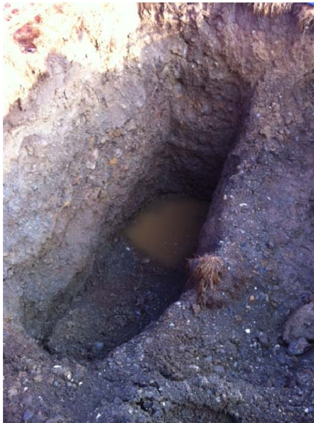
Test Pit DT-2, Note Standing Water
